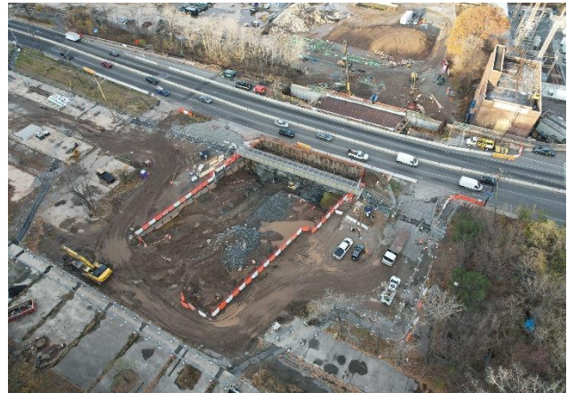
The pedestrian bridge, which provides a crossing over the construction site, opened to the public on November 27, 2024
