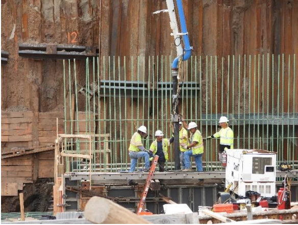
The HTP's first concrete pour took place at Tonnelle Ave. in September 2024
