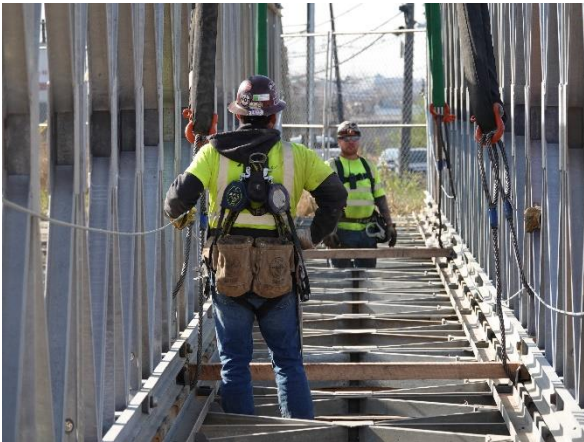
Installing the temporary pedestrian bridge on the eastern side of Tonnelle Ave. in November 2024
