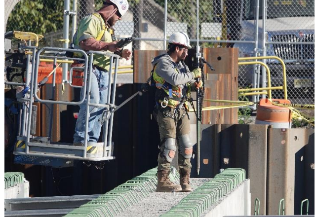
At work on beams with fortified bars that undergird the concrete deck in October 2024
