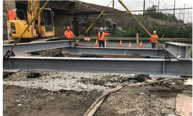
This reinforced driveway bridge will protect an 1860's-era water pipe that supplies 65% of Jersey City water
