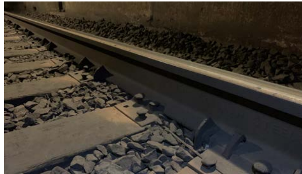
Salt Chemicals in Rock Ballast Confusing the Signal System
